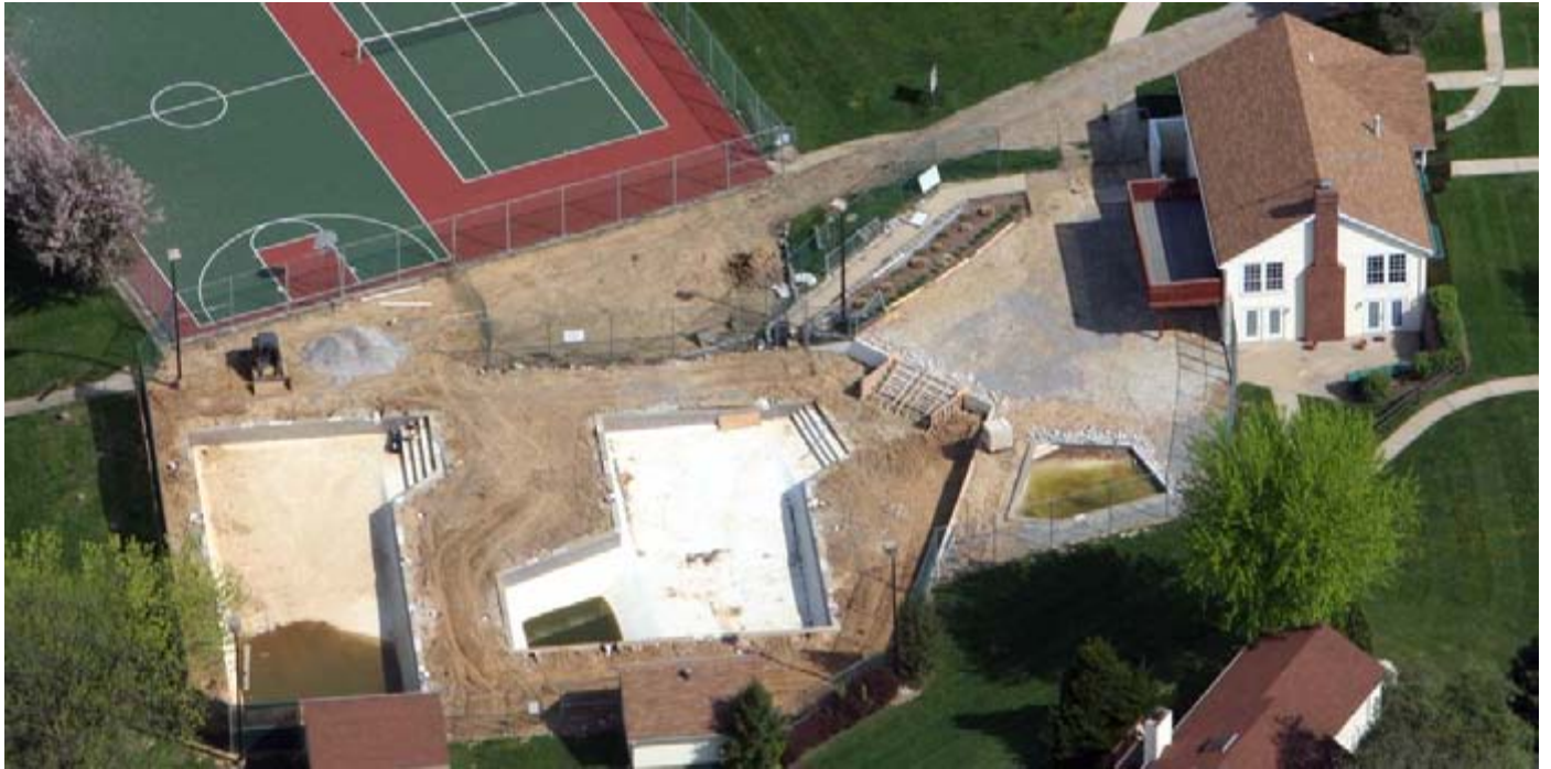
April 11, 2010; the old pool deck has been completely removed and the water lines from the pump house to the pools have been repaired.
