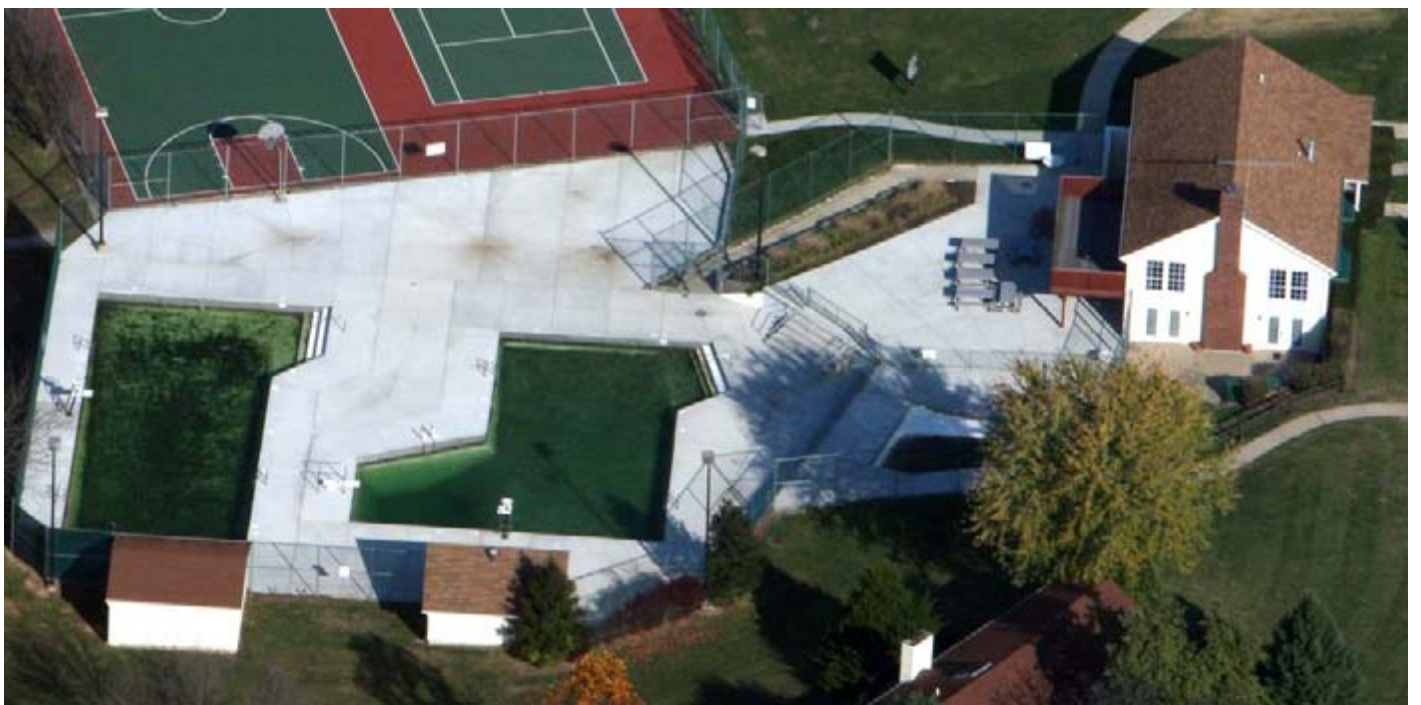
October 31, 2010; the pools have been closed for several weeks. Concrete work has been completed.
